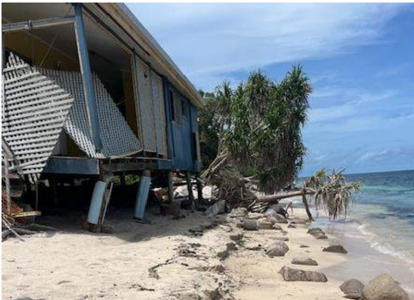
Image – Jan 2025 (note: the inclusion of defence works in this location TBC, due to current condition and safety to workers)
